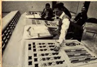
Central control panel of the Aswan scheme.
